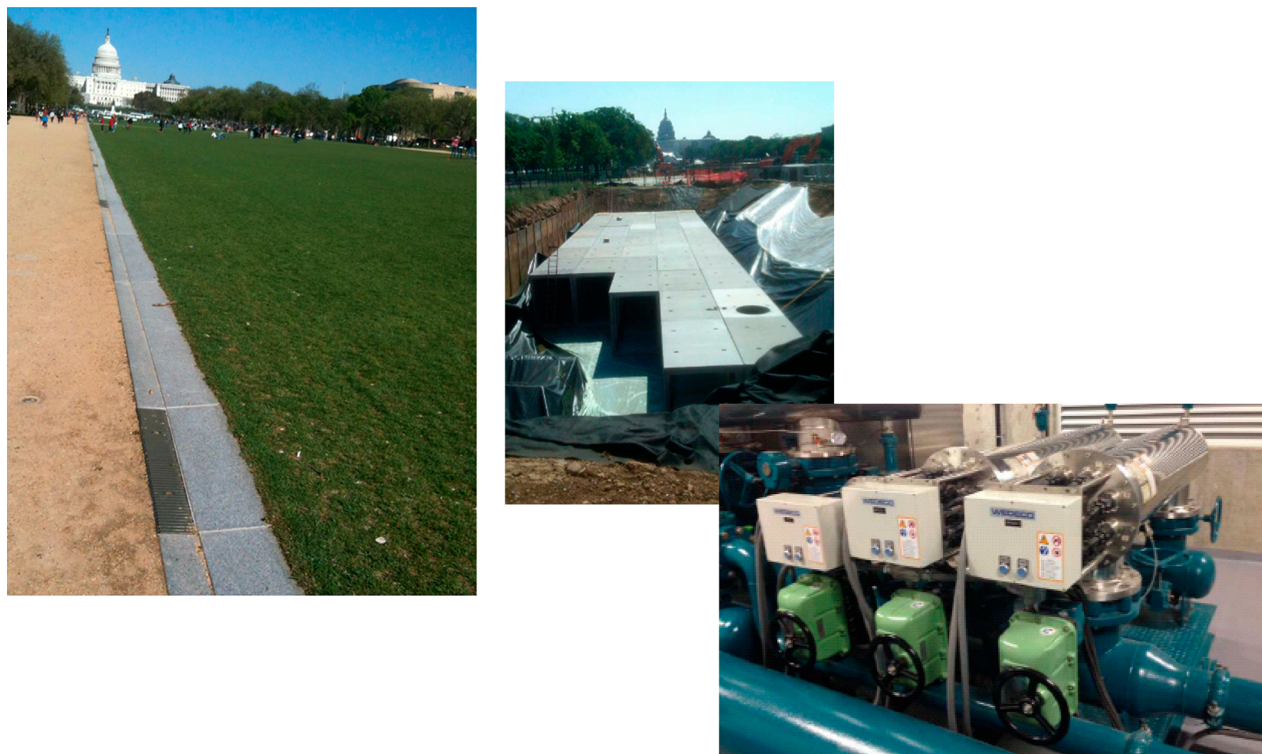
Figure 1. National Park Service constructed large stormwater cisterns under the National Mall for turf irrigation (center photo). Stormwater is processed through microscreens and ultraviolet light disinfection (right photo). On-site stormwater use is attractive where rainfall is more uniform throughout the year. (Right and left photos by the authors, center photo National Park Service).
